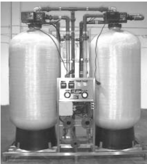
FIGURE 12: Typical Sorption System Composed of Pressure Vessels with Iron-based Sorption Media Capable of Treating 100 gpm (AdEdge Technologies, Inc., Norcross, Georgia)
