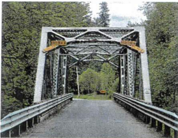
Ferrier Bridge #93 is posted with height restrictions
